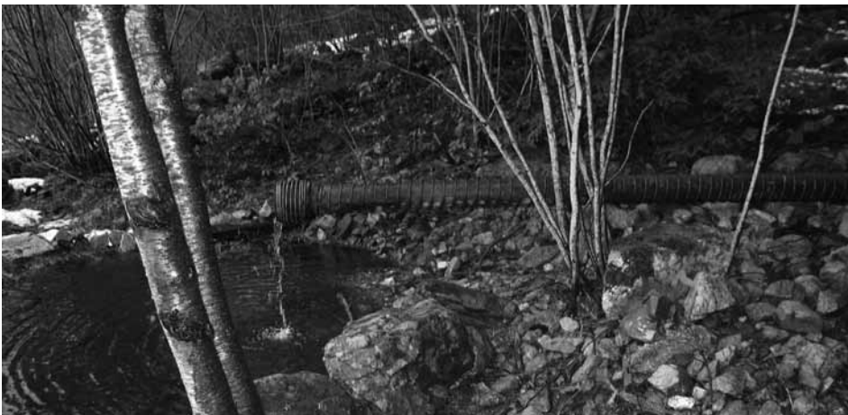
This photo shows wire-wound wood pipe still carrying water at Alexandra Lodge. Photo courtesy Lorna Fandrich
