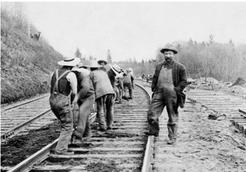
A Chinese crew working on a railroad, with a white man as Foreman. They are laying track and there are three tracks side-by-side.
